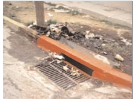
Storm drain violations as seen here, are now subject to stiff fines and penalties. The City is mounting an aggressive campaign to reduce the amount of pollutants flowing into the Santa Monica Bay (below) and surrounding coastal waters.
