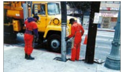
Bureau of Sanitation crews routinely clean out the City's 55,000 catch basins and step up the frequency prior to and in anticipation of the rainy season.
