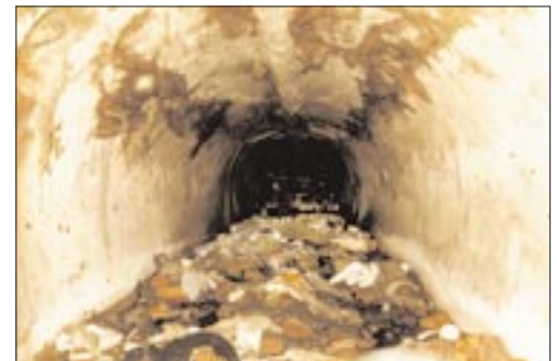
In a photo taken via remote controlled camera, trash over two feet deep blocks this underground storm drain pipe. Debris not only prevents proper drainage, but also invites unhealthy neighborhood conditions such as odors, rats, and as seen along the walls, roaches and other vermin.
