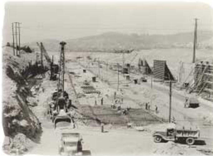
Upstream view (1939) from what is now the Pasadena Freeway showing channel work in progress.
